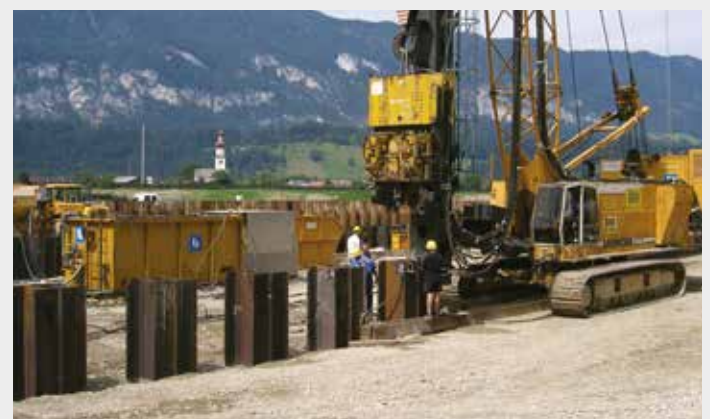
Fig. 11. Template with a single level and piling equipment guided on a fixed leader.
